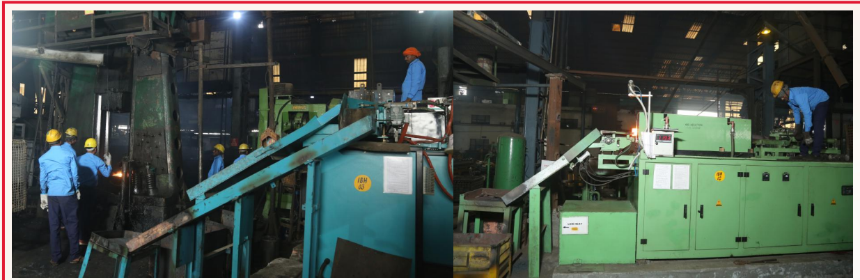
PLANT IS EQUIPPED WITH INDUCTION BILLET HEATER WITH 3 WAY MECHANISM & DUEL COLOUR PYROMETER.
